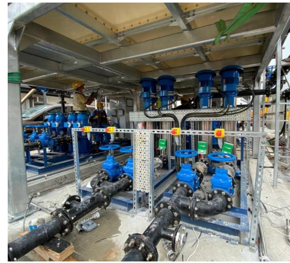
Installed Pump Modules
