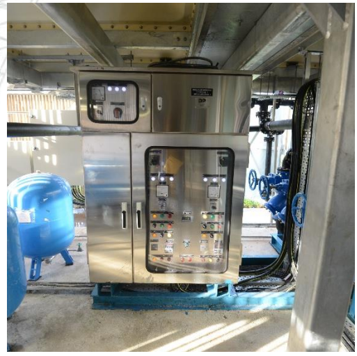
Installed Electrical System and Control Panel
