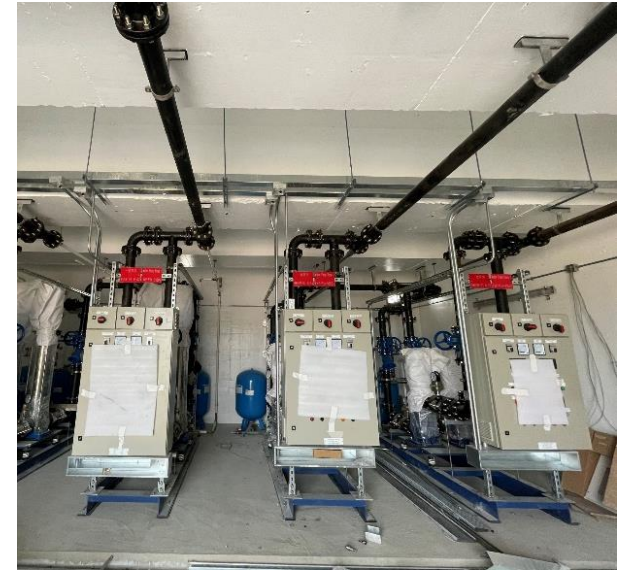
Pump Room Electrical Panels and Pump Modules
