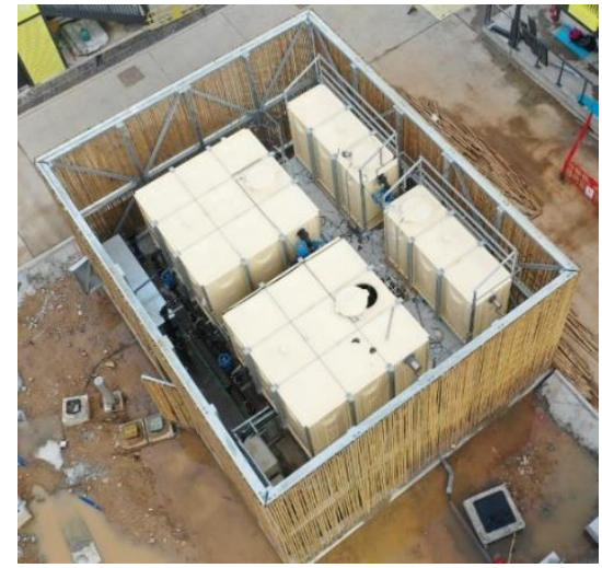
Birds-eye View Of Installed Pump Room
