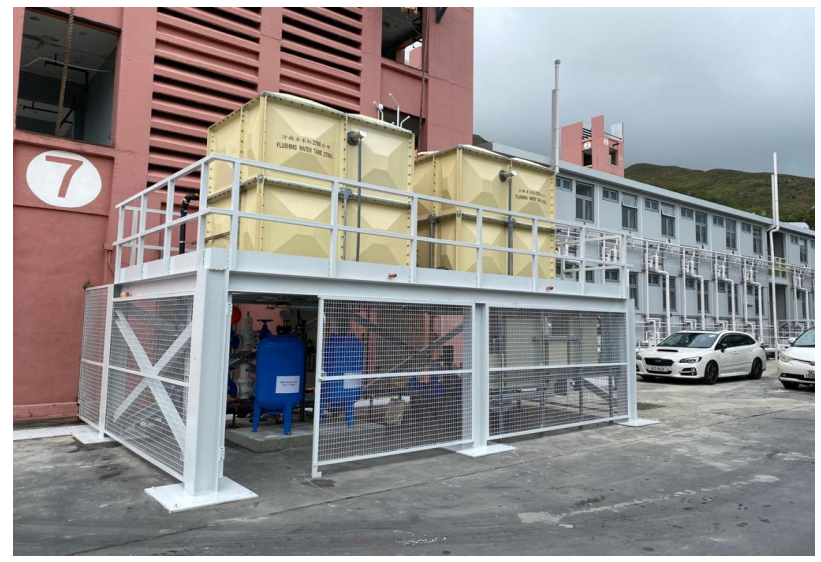
Pump room modules in Pat Heung
