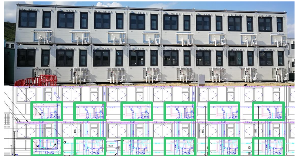
Actual Installed Modules and BIM Drawing of Drainage Module Installations for Pre-alignment
